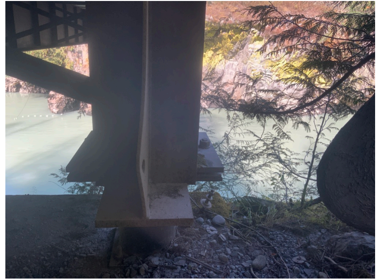
Jump span bearing. Upstream. Deformation
